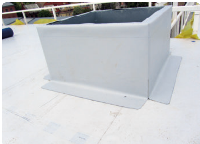
Tooling of skylight / smoke flap
