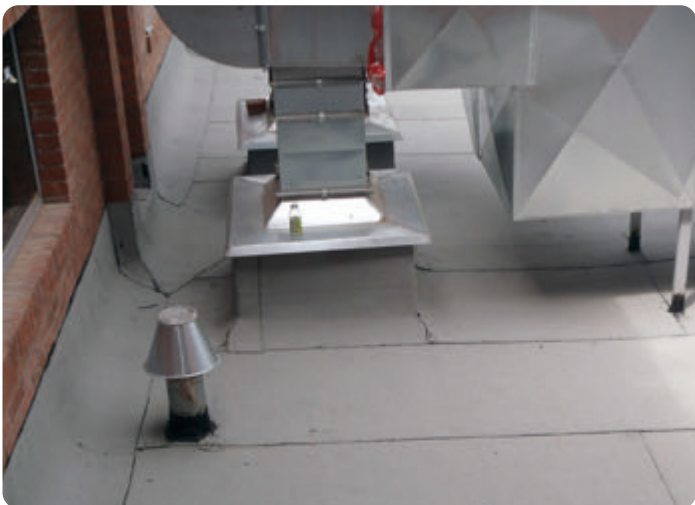
Access to ventilation equipment
